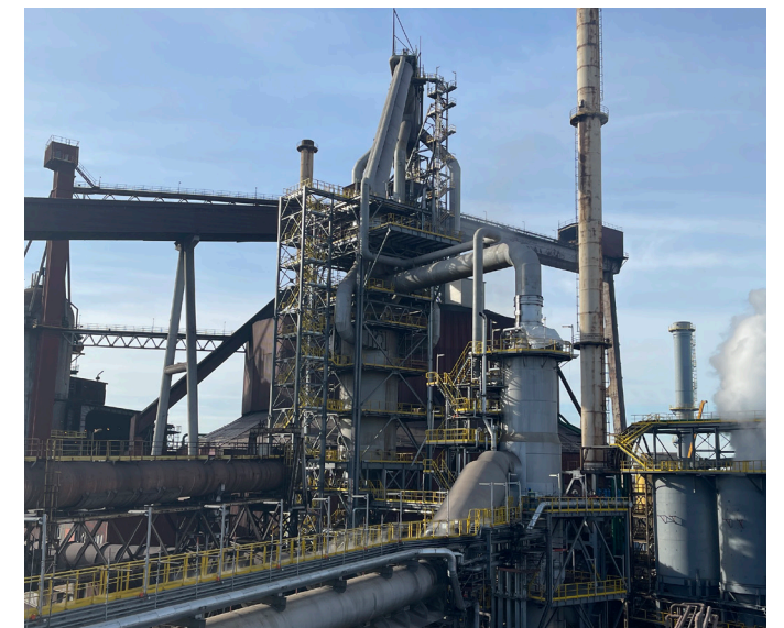
New off-gas system and gas cleaning plant
