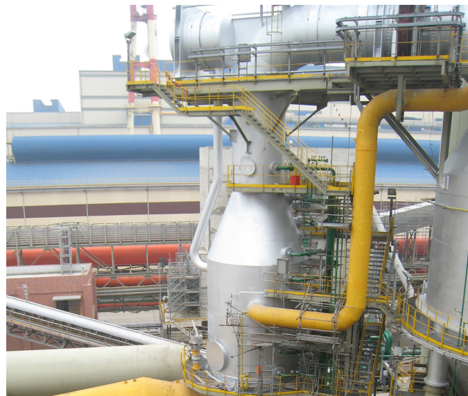
Gas cleaning plant at Dragon Steel BF 1
