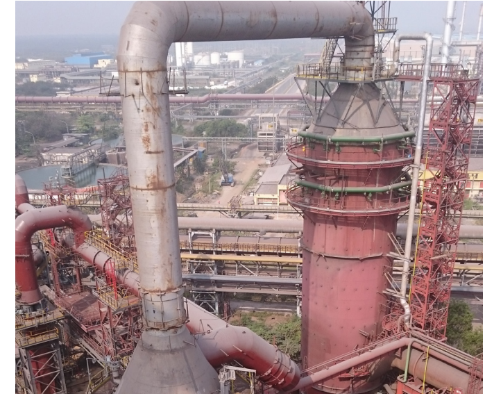
New Davy Cone Scrubber installed inline with existing spray tower
