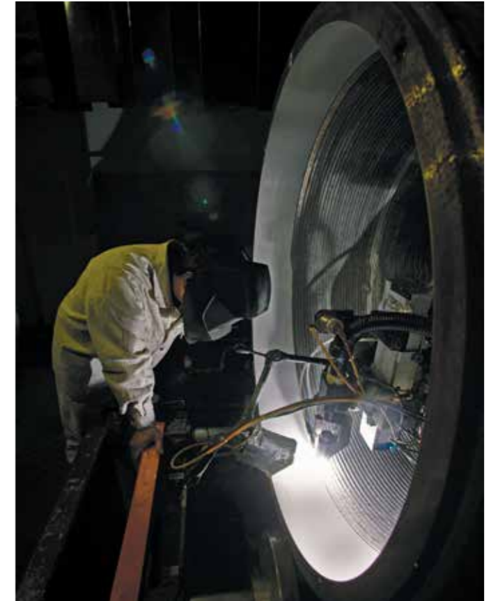
High Strength Babbitt welding process
