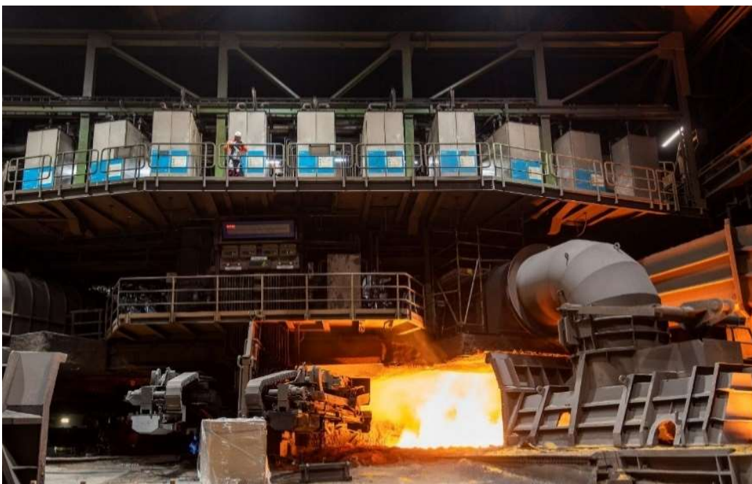
Oxygen SIP technology installed at thyssenkrupp Steel Europe, Schwelgern – blast furnace No. 1.
