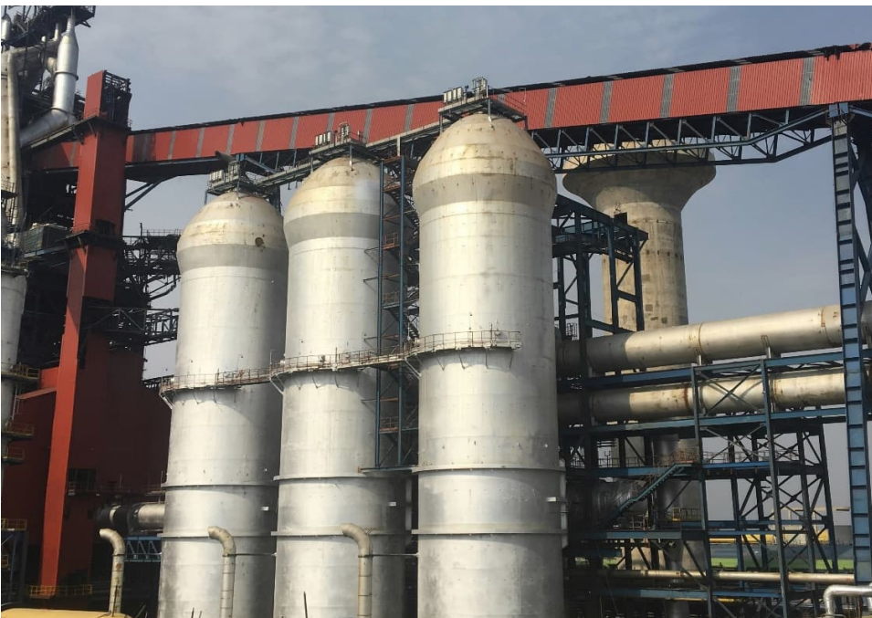
Internal combustion stoves from Primetals Technologies installed in India.
