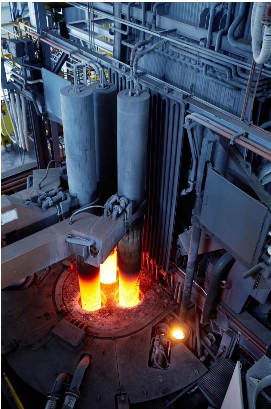
EAF Quantum electric arc furnace from Primetals Technologies
