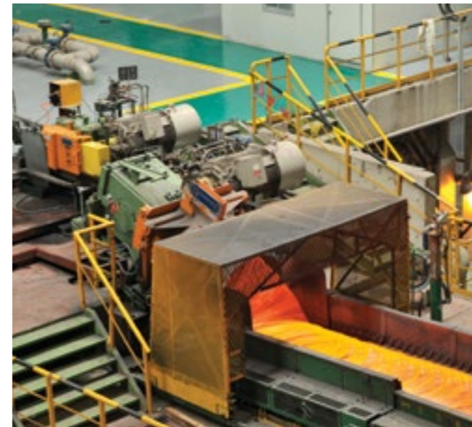
Morgan High Speed Pinch Roll and Laying Head arrangement
