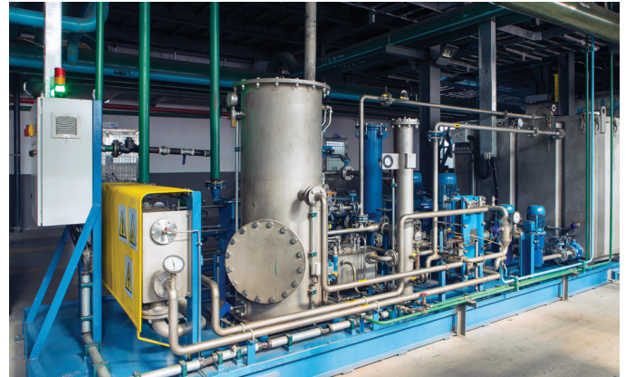
Lubrication system with vacuum dehydration
