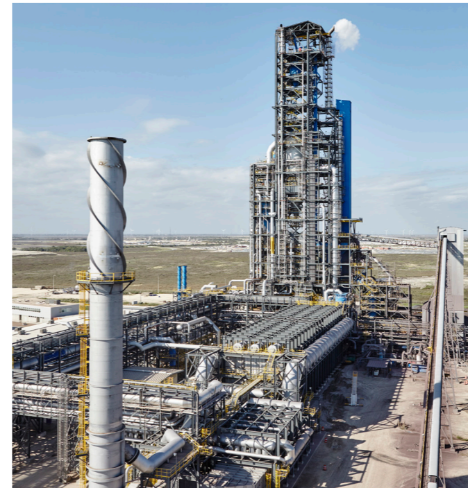
HBI plant tower and reformer
