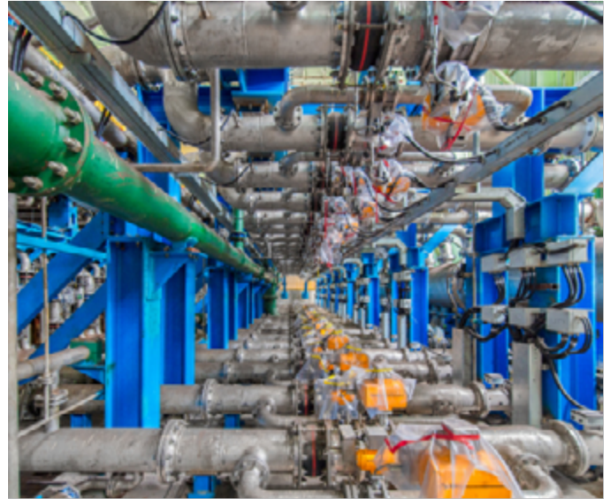
MULPIC intermediate pipework
