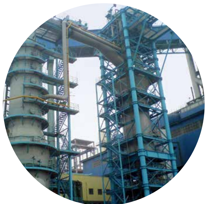
Xianghan blast furnace conditioning tower and scrubber
