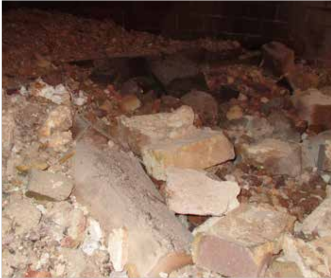
Damaged internal stove
