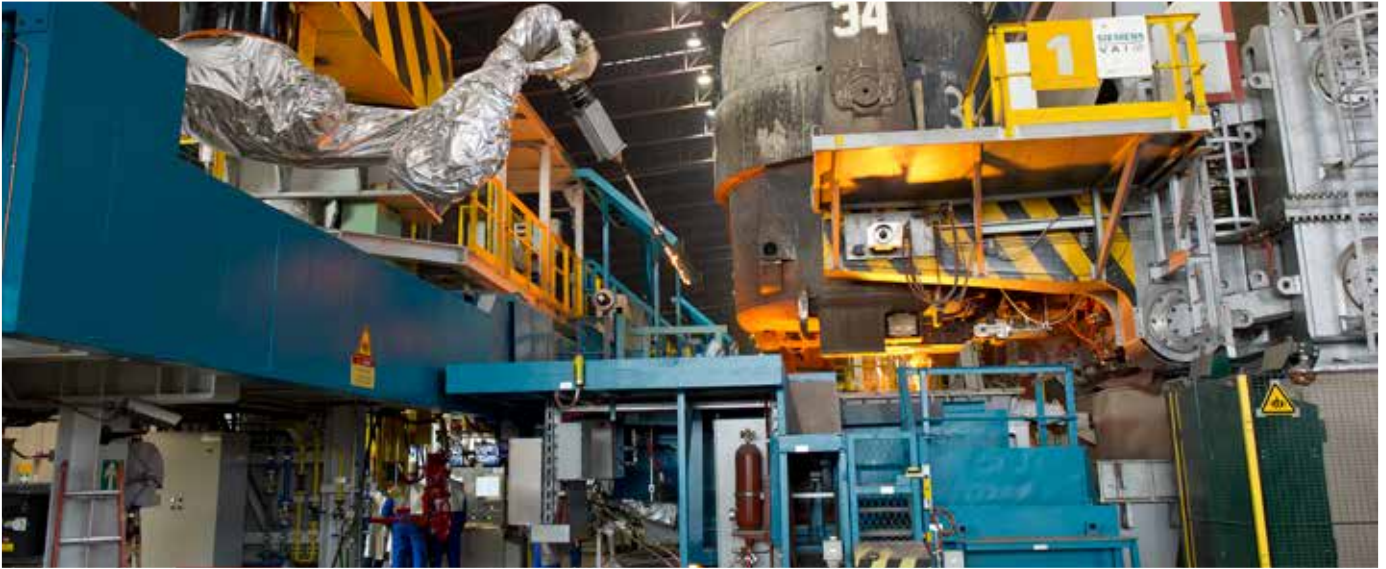
Single strand slab caster, voestalpine Stahl, Linz, Austria
