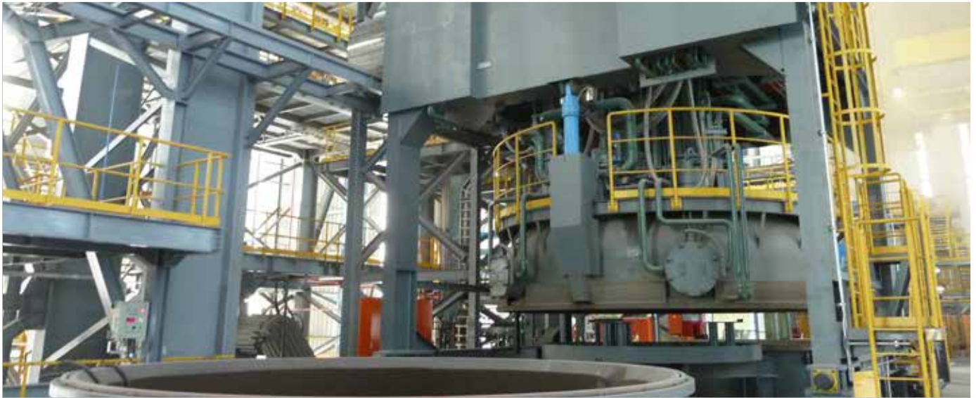
Efficient layout and modern dry mechanical vacuum pumps can make the VD highly profitable
