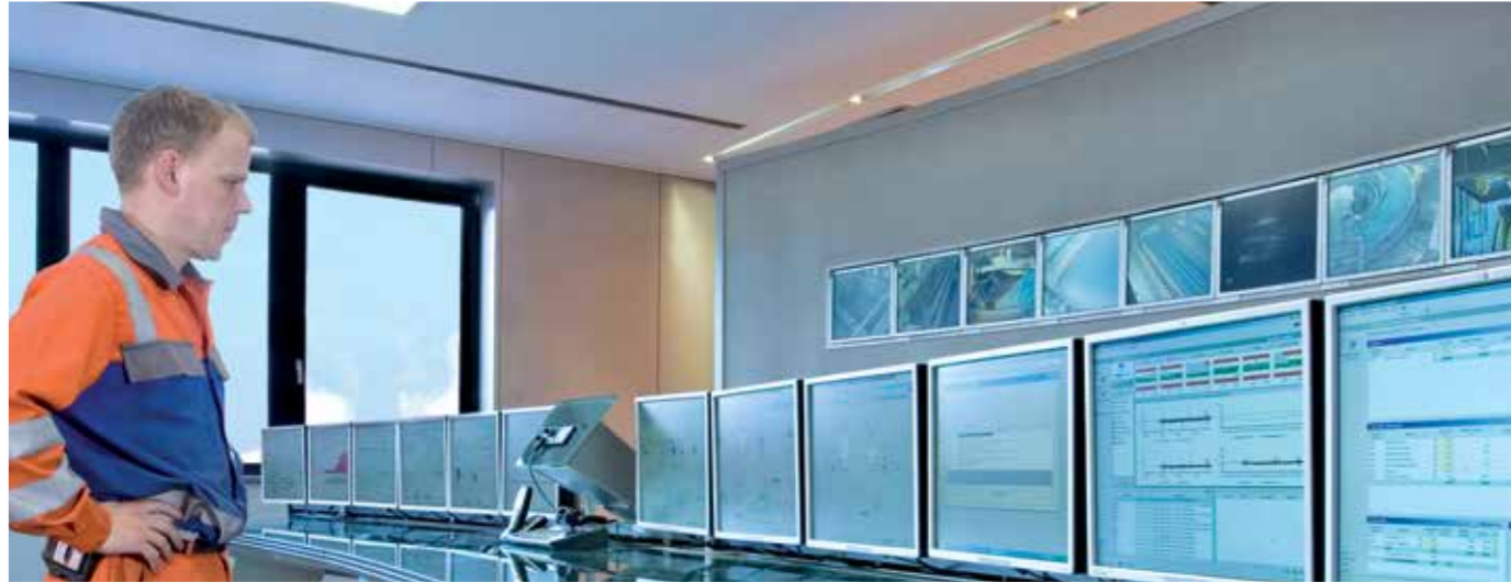
Sinter plant control room, voestalpine Stahl GmbH, Linz, Austria
