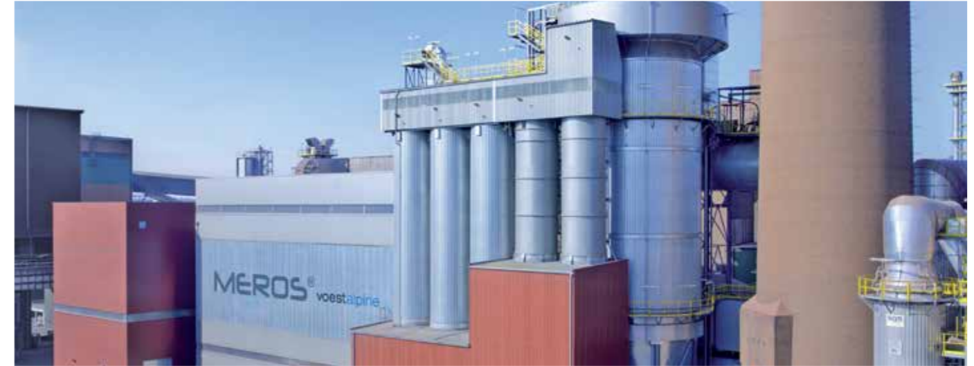
MEROS plant voestalpine Stahl, Linz, Austria
