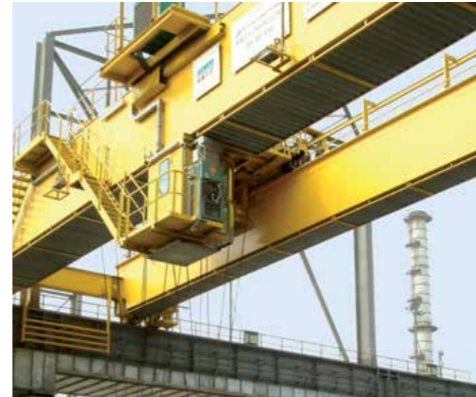
Slab handling crane, suited for hot slabs up to 850° C
