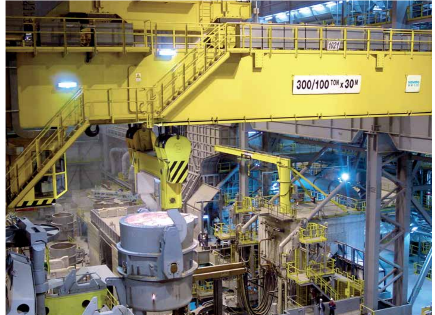
Teeming crane, stainless steel meltshop
