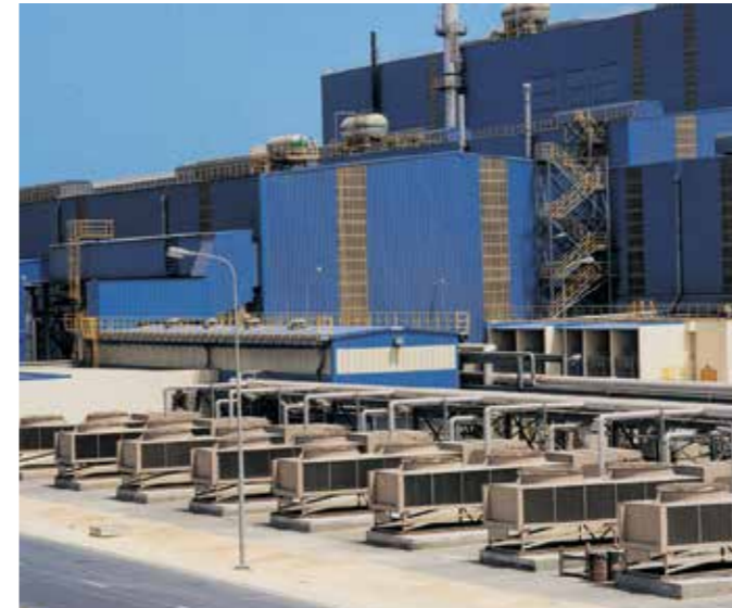
Chiller units for air conditioning
