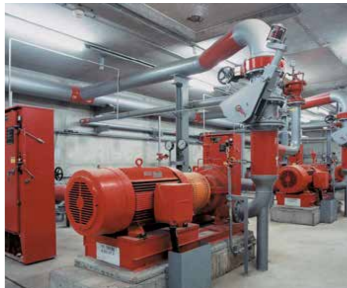
Fire fighting pump station
