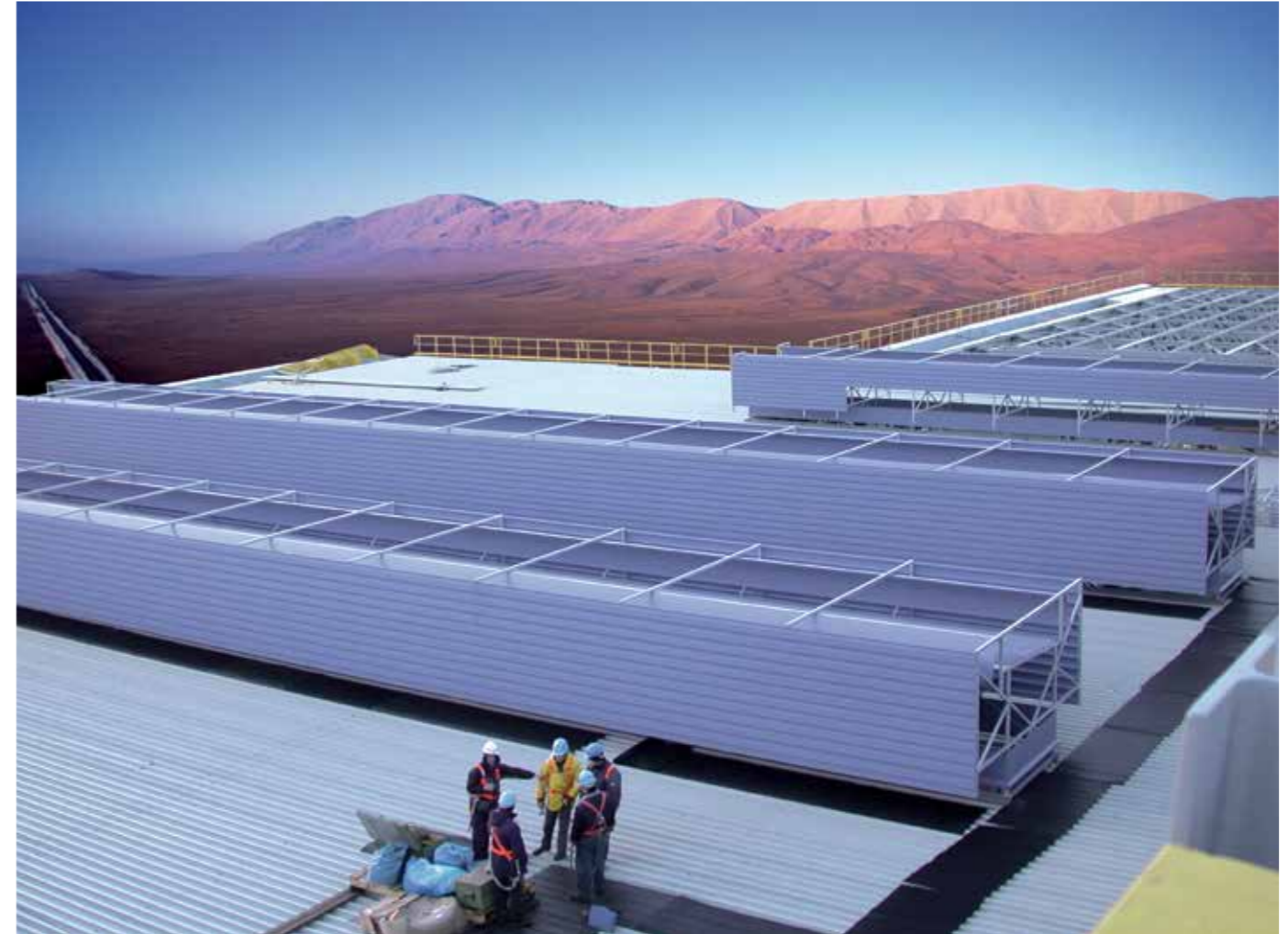
Roof ventilator for natural ventilation
