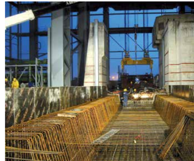
Converter foundation - emergency pit
