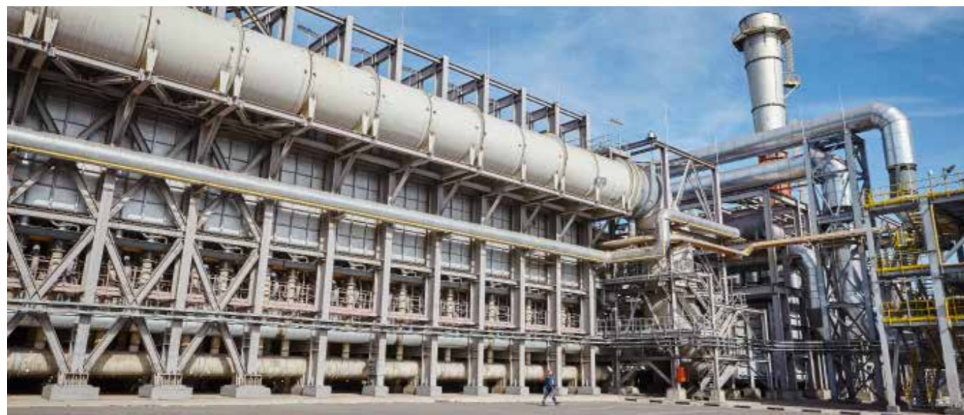
The reformer, transforming natural gas to reduction gas
