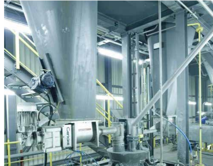
Additive dosing station
