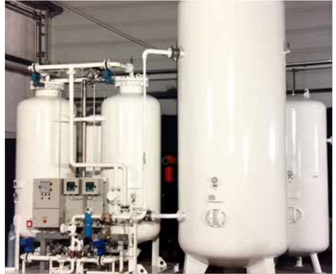
Nitrogen generator (nitrogen purity: 99,9 vol%)
