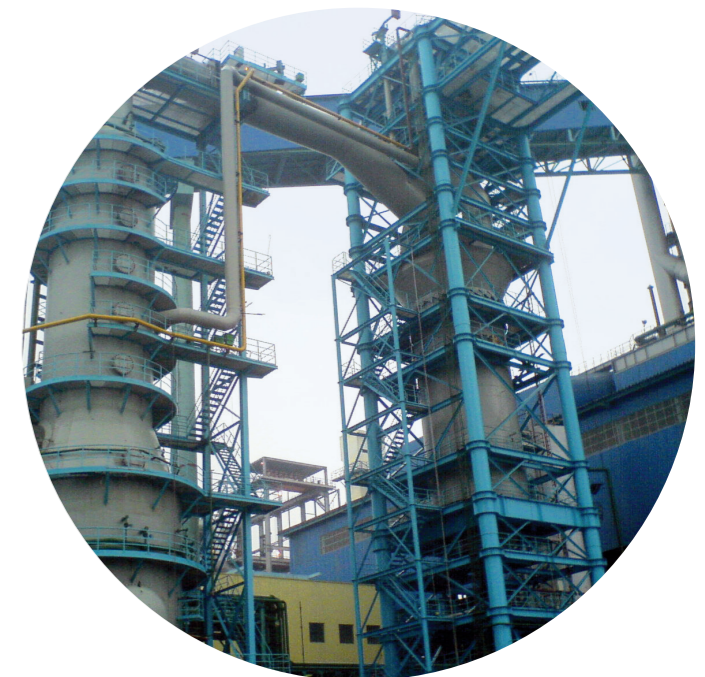
Xianghan blast furnace conditioning tower and scrubber
