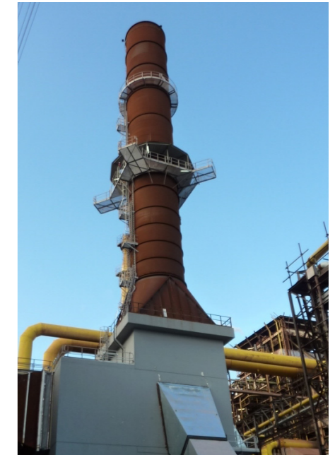
Secondary dedusting system at one of the sinter plants of Ilva S.p.A. in Taranto, Italy
