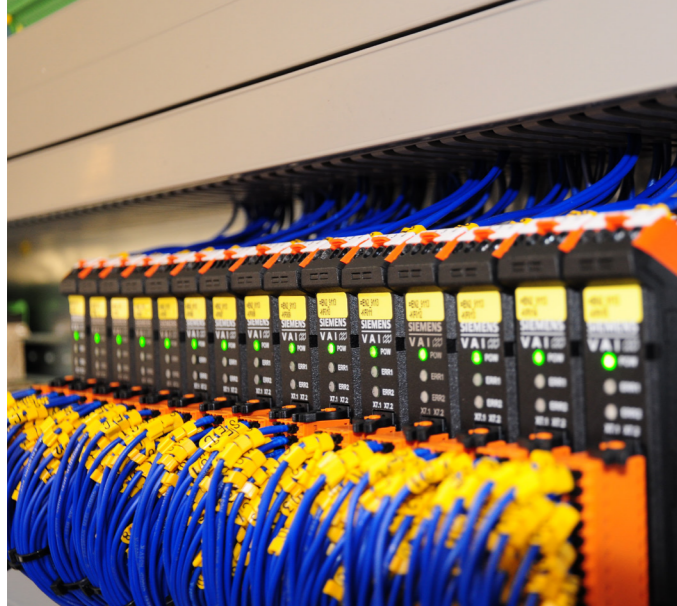
Electronic modules of the bag filter units
