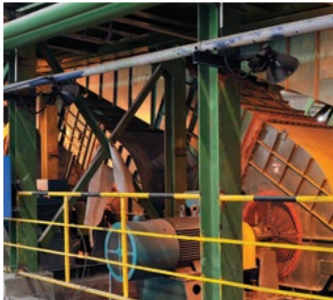
Fans located beneath the Morgan Stelmor Conveyor
