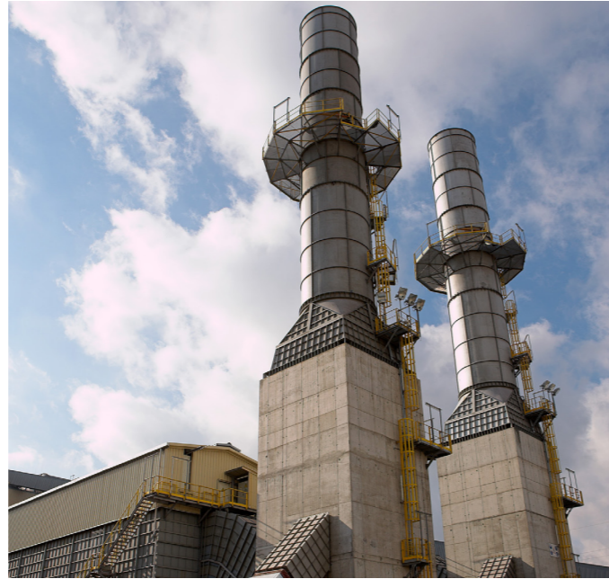
Bag filter plant with stack
