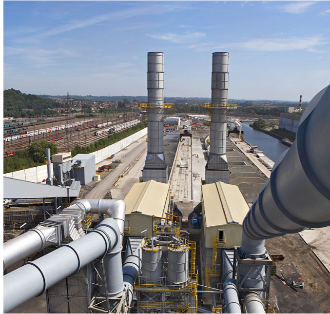
Primetals Technologies dedusting plant
