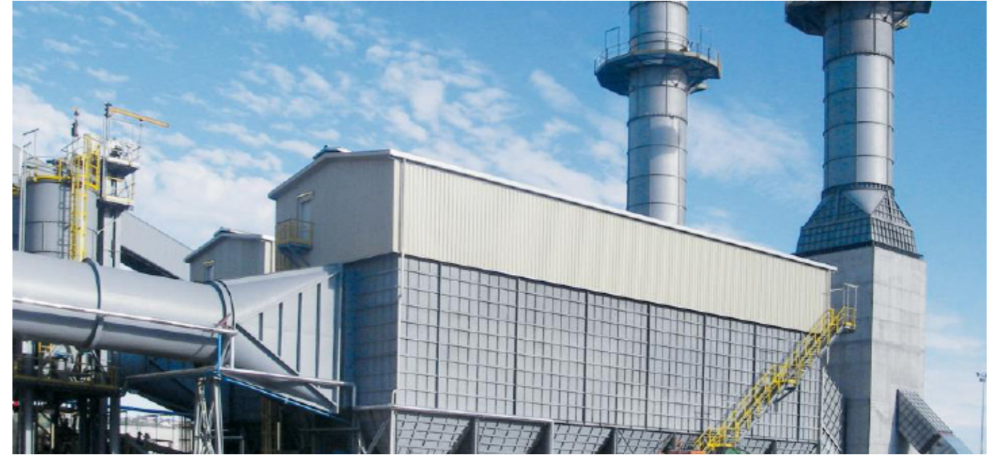
EAF dry dedusting system bag filter plant and stack
