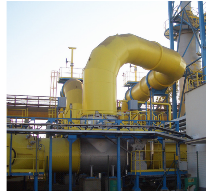
Switch-over station for wet-type dedusting
