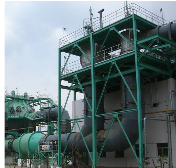
Switch-over station for dry-type dedusting
