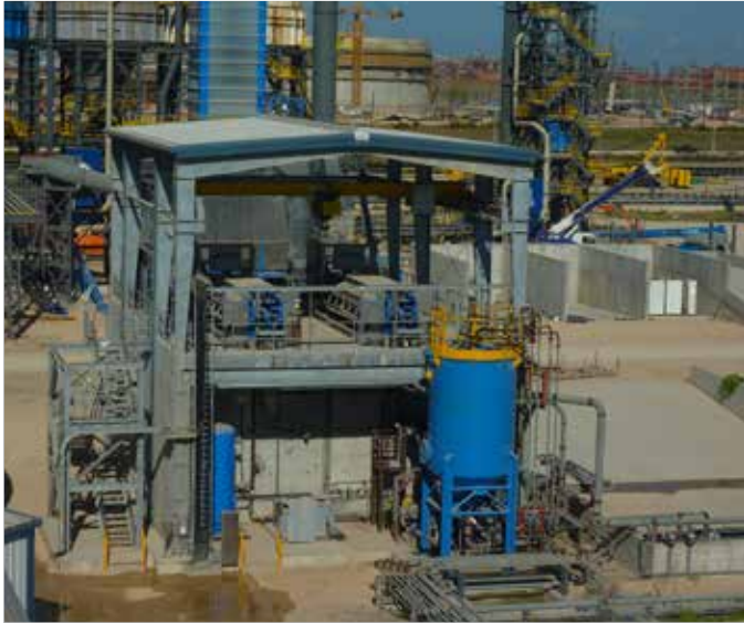
Fig. 2: Slurry treatment with the dewatering unit
