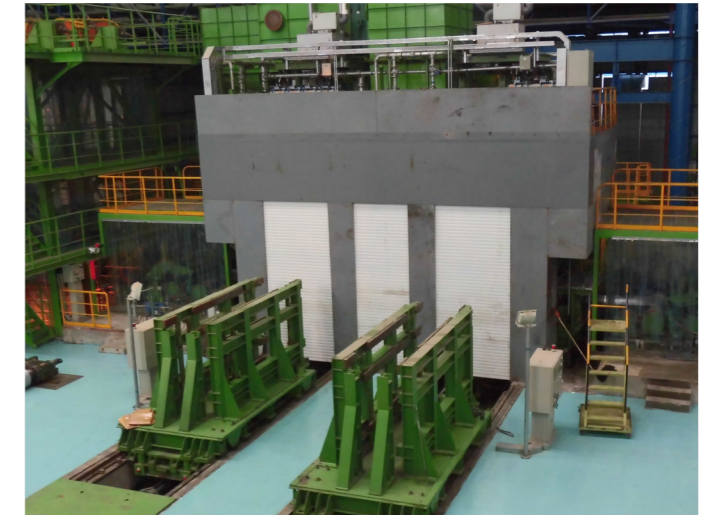
Temper mill, WIN Steel, Wuhan, China
