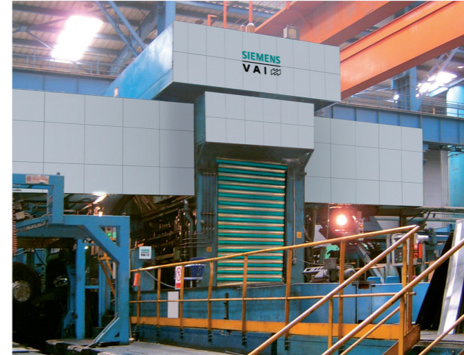
Reversing cold mill, Tangshan Iron & Steel, Tangshan, China
